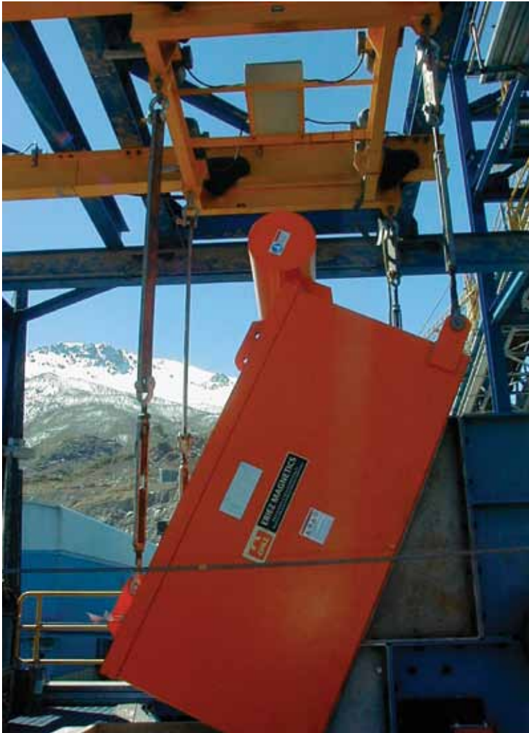
An installed Eriez magnetic separator.
